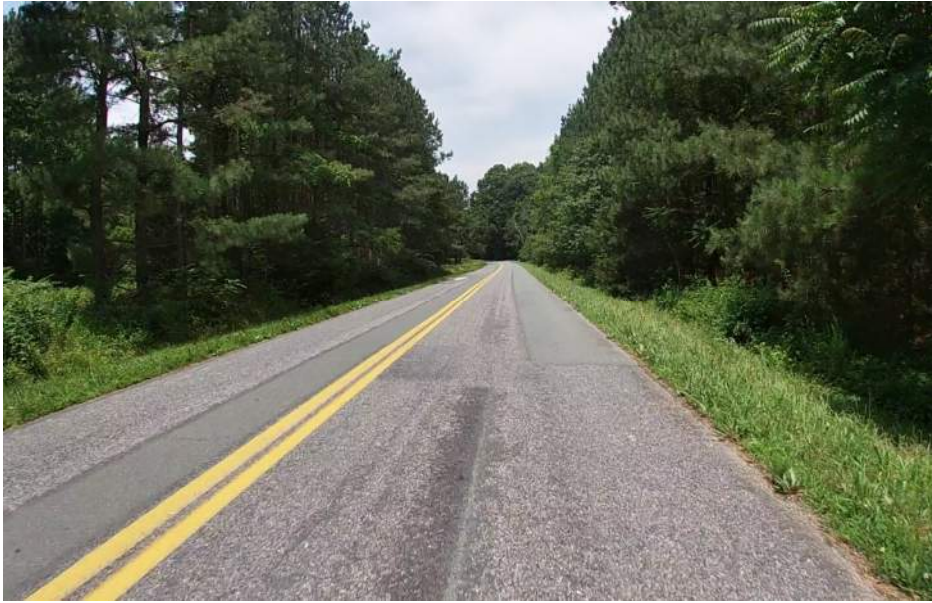
8. Block Cracking, Patching
