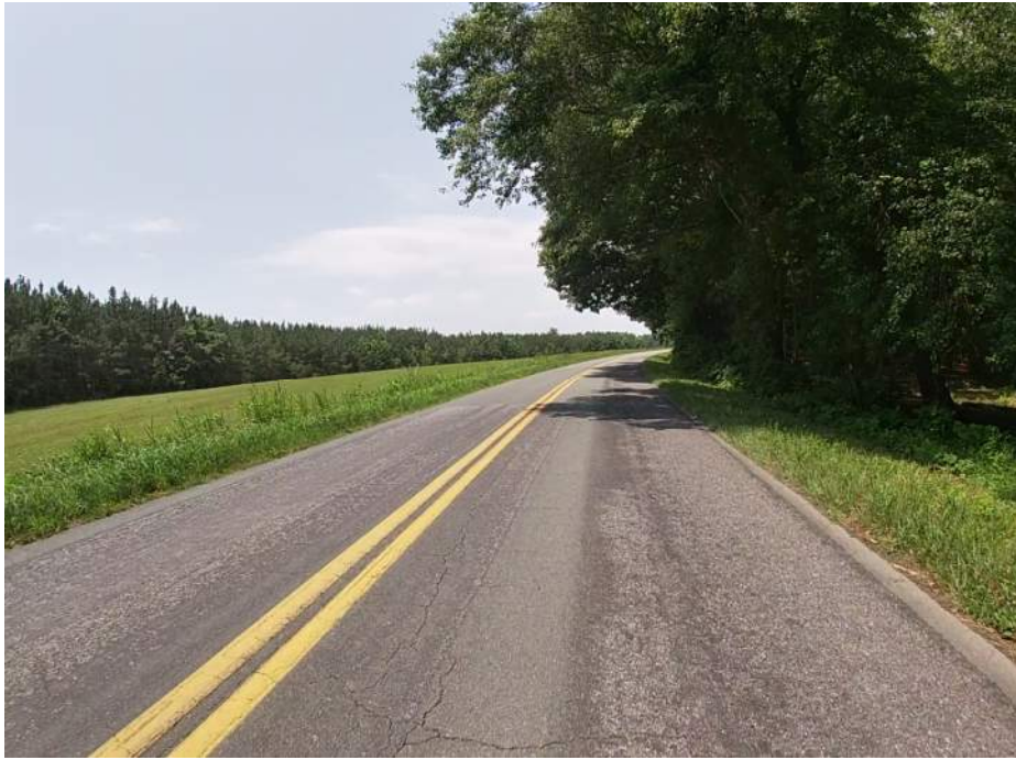
6. Block Cracking, Patching
