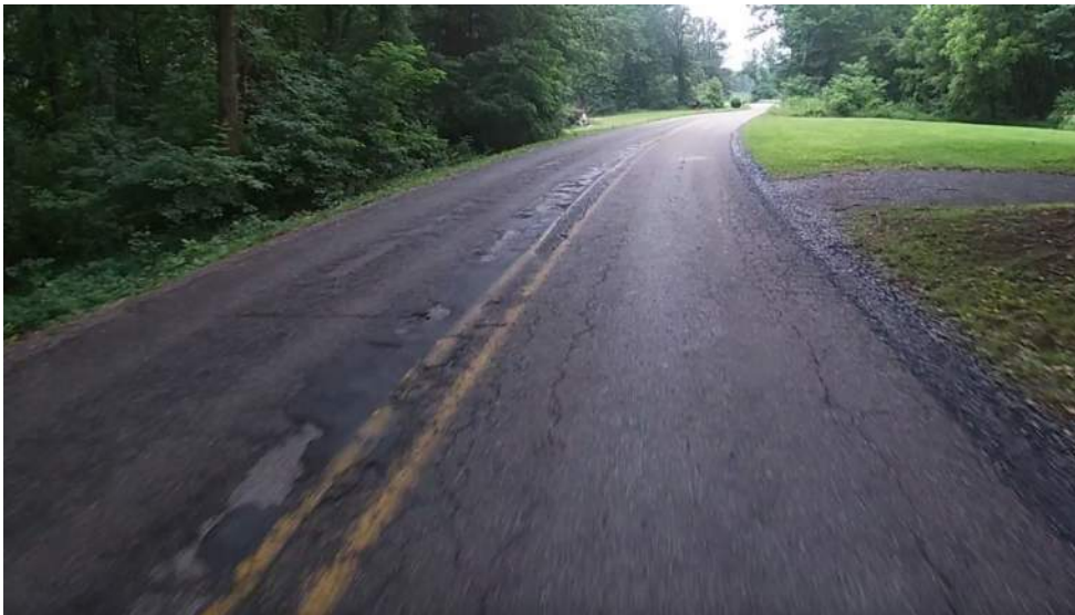
6. Patching and Potholes
