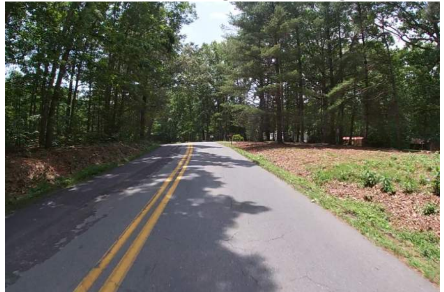
22. Block Cracking, Patching
