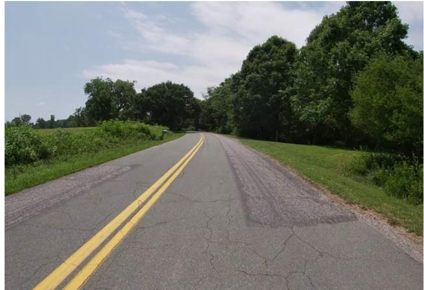
14. Block Cracking, Patching
