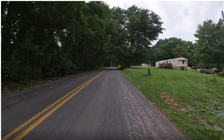
49. Alligator Cracking, Patching
