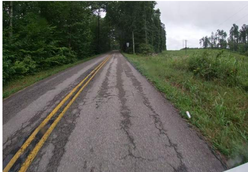
20. Patching and Alligator Cracking
