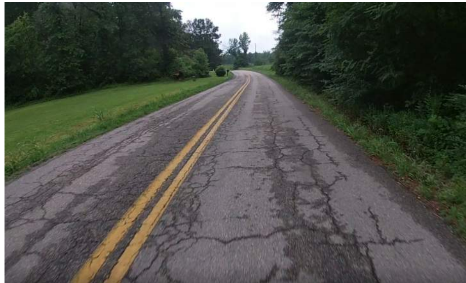
10. Patching and Edge Raveling
