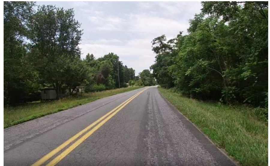
18. Block Cracking, Patching
