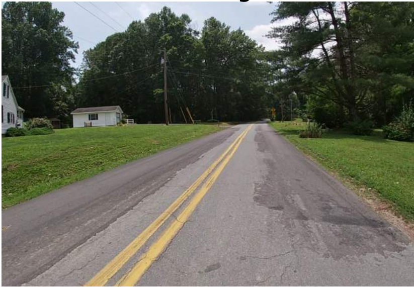
21. Block Cracking, Patching
