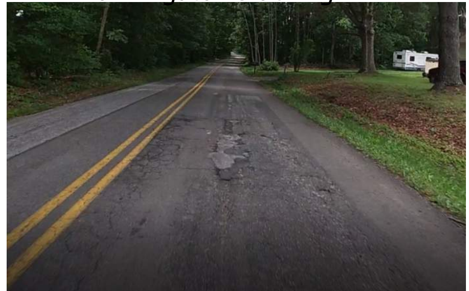
42. Patching, Alligator Cracking
