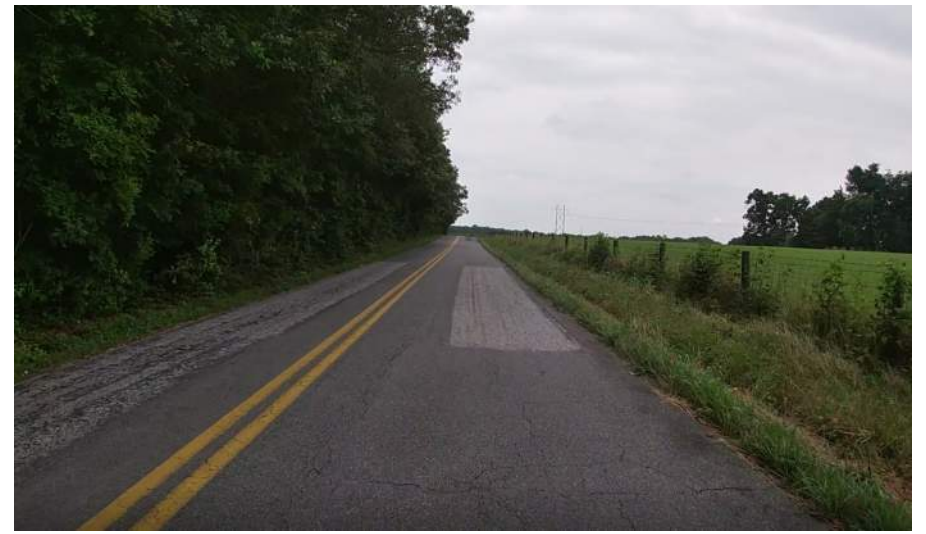
32. Alligator Cracking, Patching
