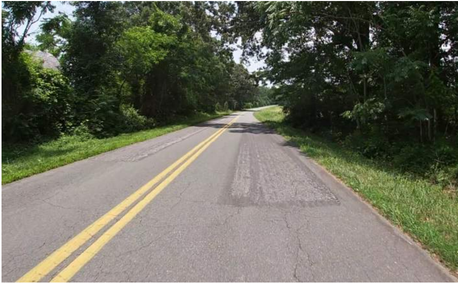
15. Block Cracking, Patching
