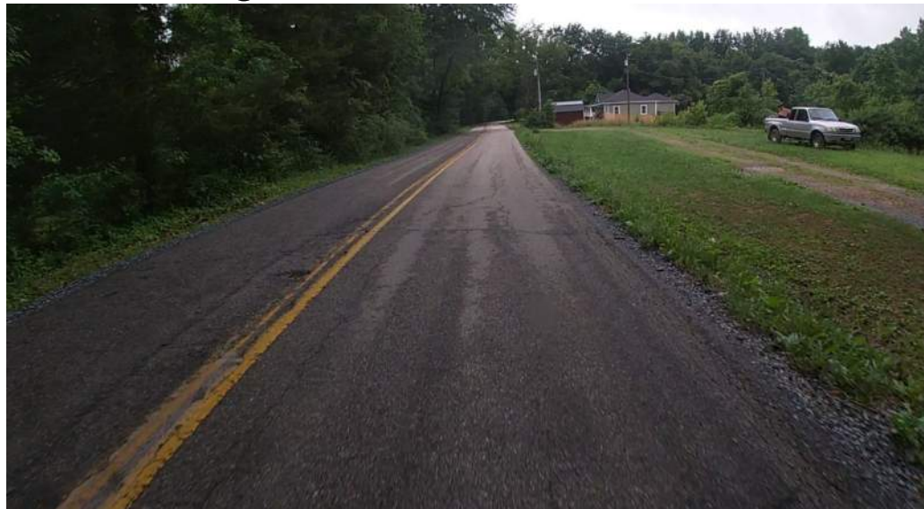
3. Patching and Edge Raveling
