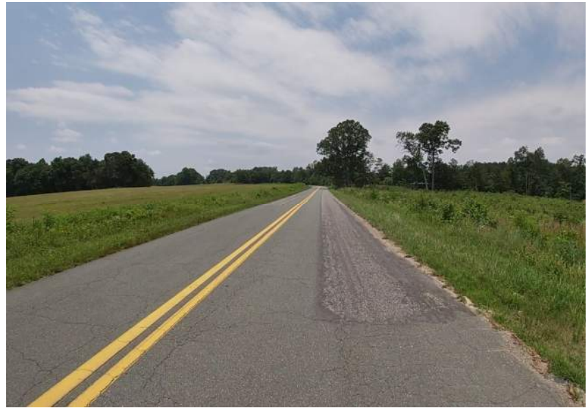
12. Block Cracking, Patching
