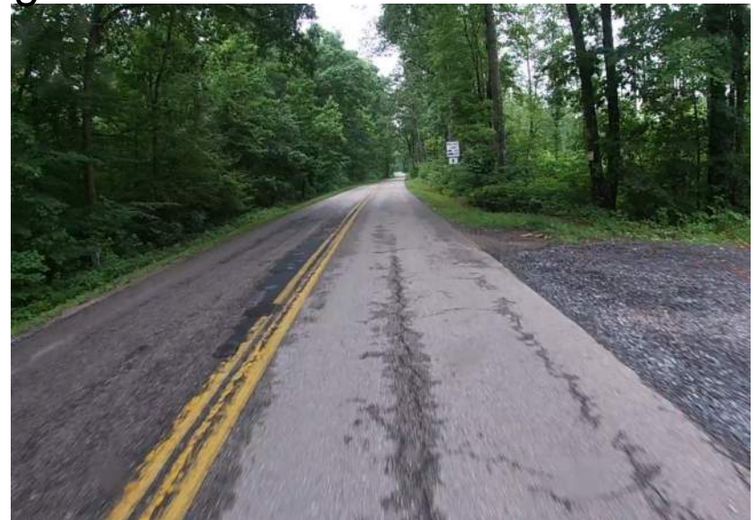
21. Patching and Block Cracking
