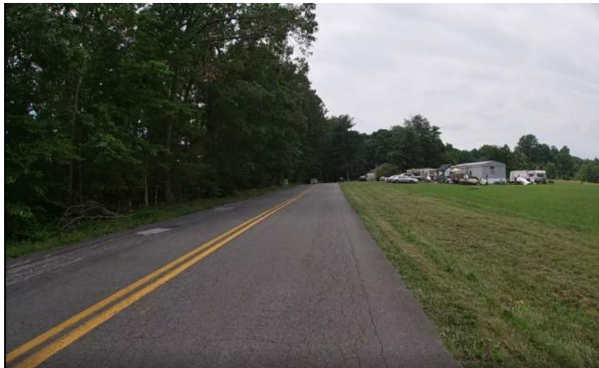
41. Patching, Alligator Cracking
