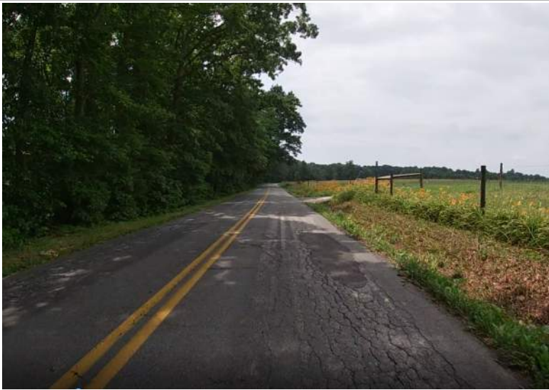
39. Patching, Alligator Cracking
