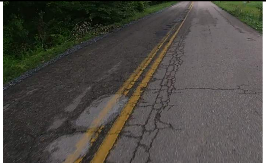
5. Patching and Block Cracking
