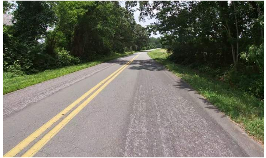
16. Block Cracking, Patching
