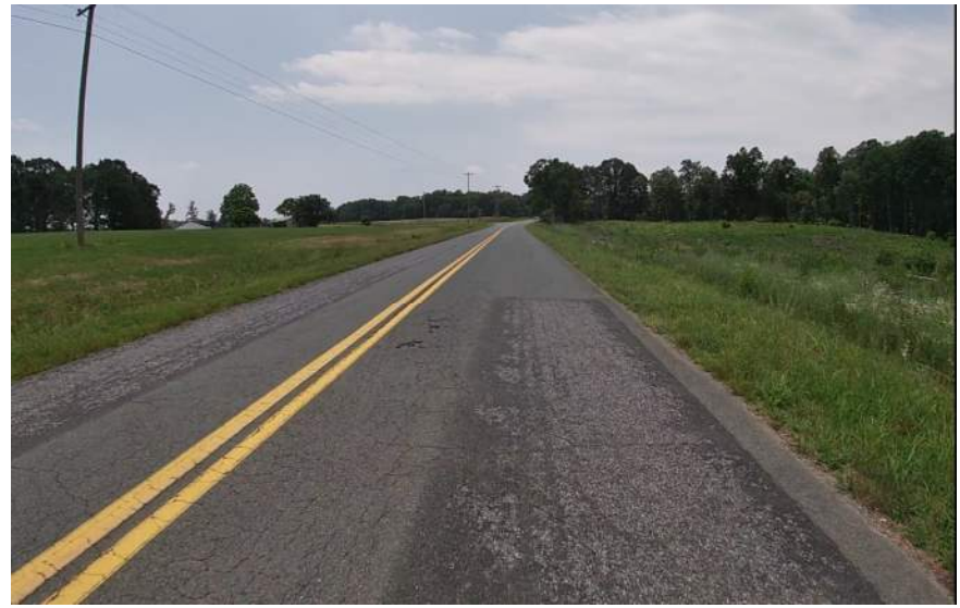
20. Block Cracking, Patching
