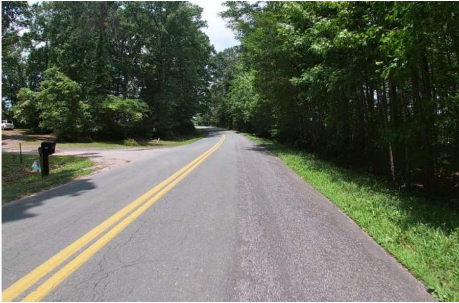
11. Block Cracking, Patching
