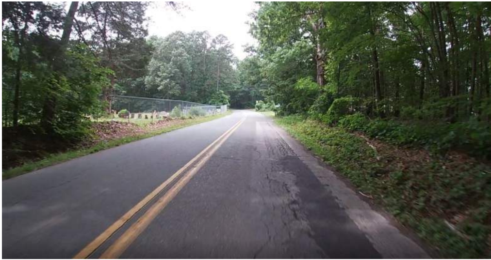
47. Alligator Cracking, Patching
